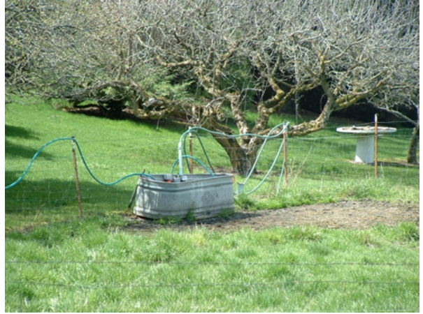
How effective is your cross-connection control program?
